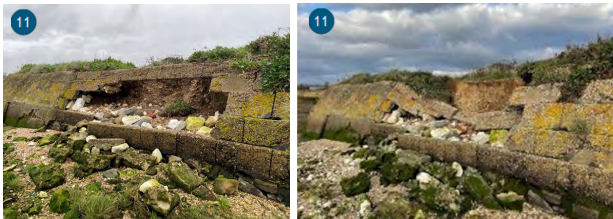
Figure 4-1 Left image shows condition of the coastal defence in November 2022 and right image is the same section of defence in January 2023
