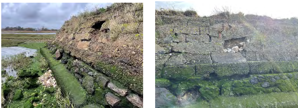
Figure 4-2 Emerging zones of weakness along the coastal defence that are more susceptible to deterioration (courtesy of Uwe Dornbusch)
