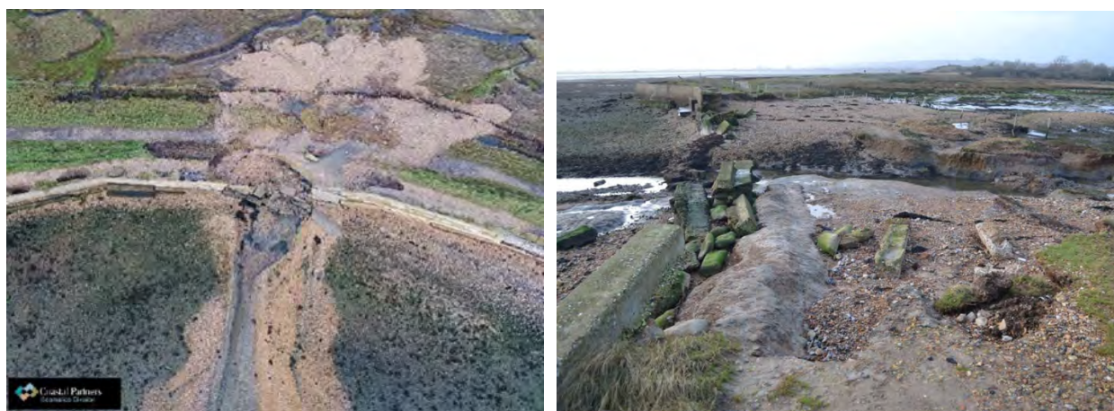
Figure 8-1 Left: Aerial photography of the unmanaged breach at Southmoor (Coastal Partners 2021). Right: Photograph of breach taken during January 2023 (courtesy of David Brew)
