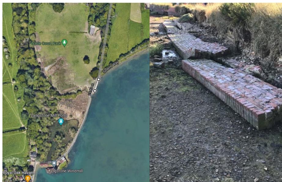
Location of failing sea defence at Langstone along coastal path (length approx.. 33m)
